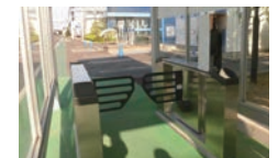
Body temperature checking system at entrances
