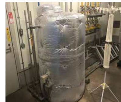
Tank covered with a thermal insulation jacket
