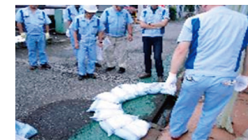
Nanno Plant: Measures against raw material leakage
