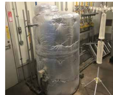
Tank covered with a thermal insulation jacket
